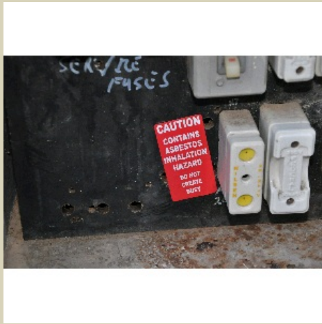
114 Asbestos Power Boards .jpg
