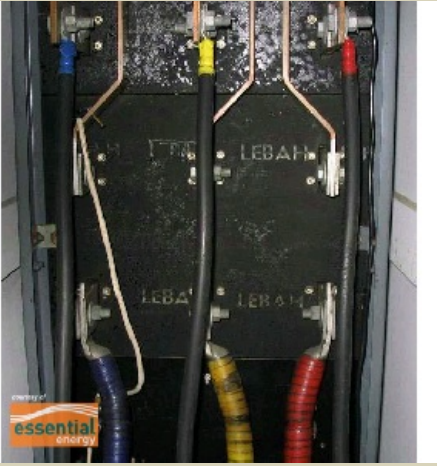
LV Distribution Board.jpg
