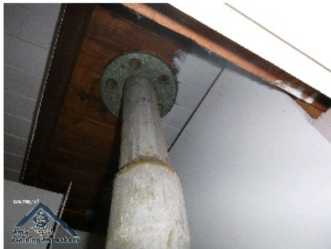
Vent pipe service cupboard3.jpg
