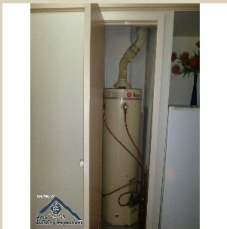
Vent pipe service cupboard2.jpg
