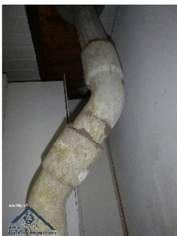
Vent pipe service cupboard1.jpg
