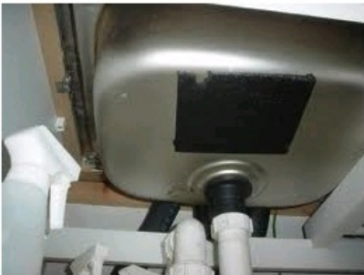
asbestos bitumen undersink.jpg
