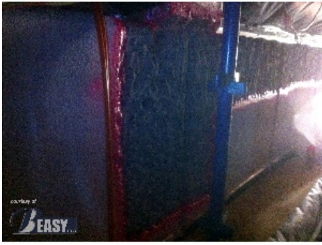
Asbestos In Cement Render_0995.jpg
