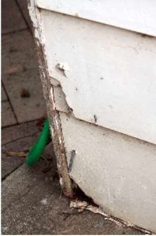
Asbestos Location - broken cladding_5973.jpg
