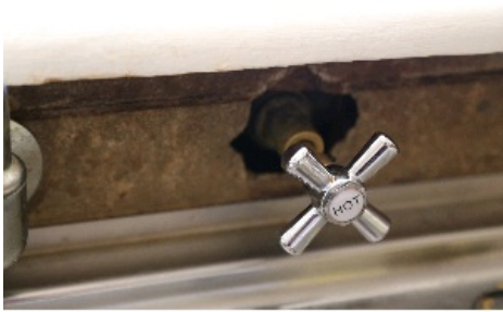
Unpainted Damaged Asbestos Cement Splashback 046.JPG
