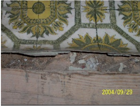
asbestos paper under lino.jpg
