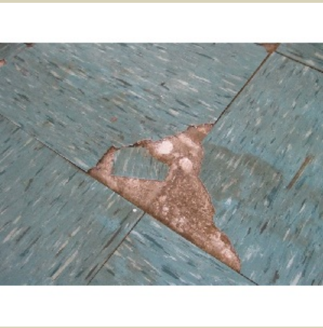
Vinyl floor tiles damaged - photo courtesy of Townsville Asbestos.jpg
