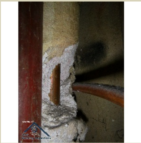
Pipe lagging service cupboard2.jpg
