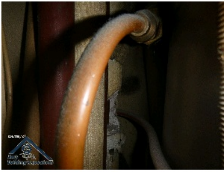
Pipe lagging service cupboard1.jpg
