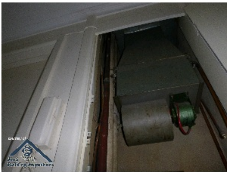
Pipe lagging service cupboard3.jpg
