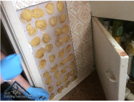
Sheeting behind tiles 2.jpg
