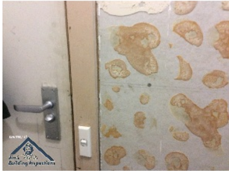
AC Wall behind tiles.jpg
