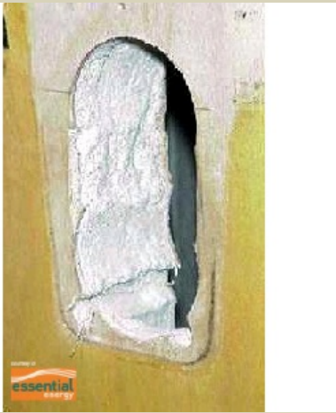
Substation Fire Doors - 2.jpg
