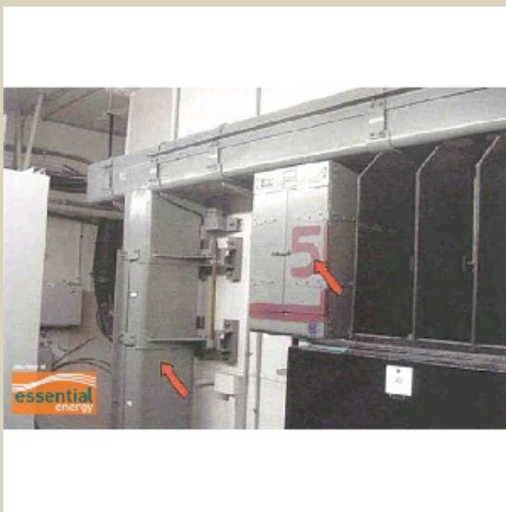
Fuse Cabinets and Busbar Trunking 2.jpg
