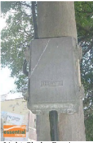
Street Light Choke Box.jpg
