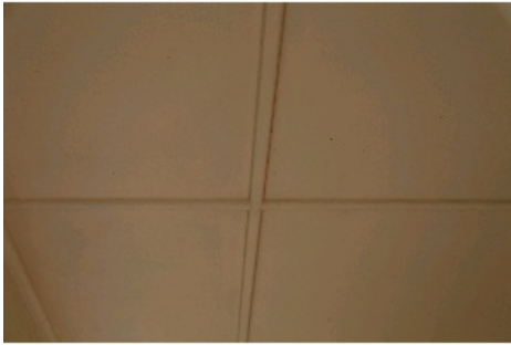
Internal Ceiling 2550 Courtesy Asbestos Awareness.JPG
