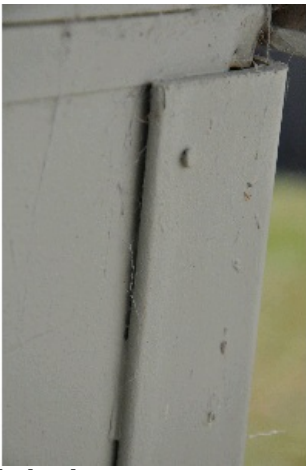
Moulded asbestos corner capping731.JPG
