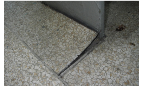
Vinyl Flooring with Asbestos
