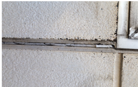
Asbestos Containing Grout
