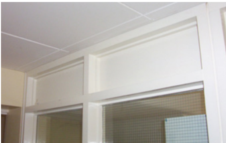
AIB Ceiling and Fire Breaks
