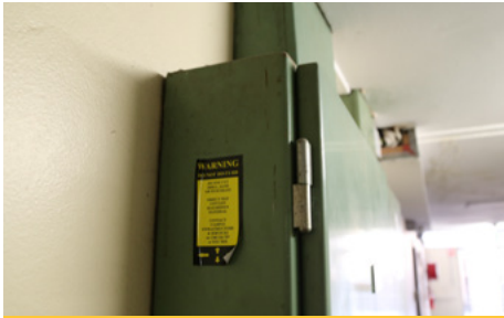
Electrical Switch Board
