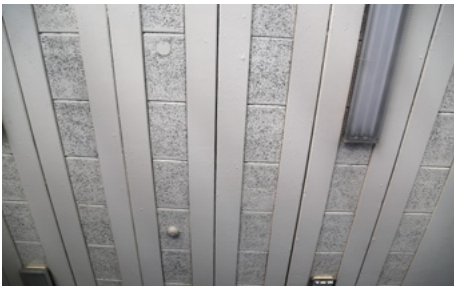
Asbestos in Ceiling
